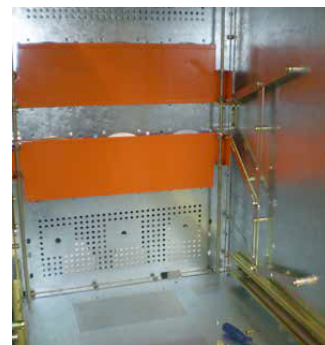
Metallic partitions (PM) between compartments for safe maintenance work.
